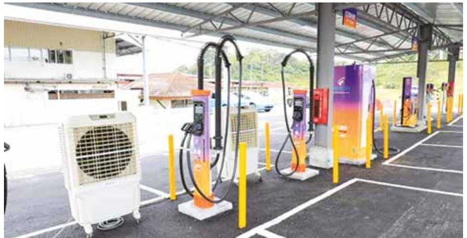
EV Charging Station.
