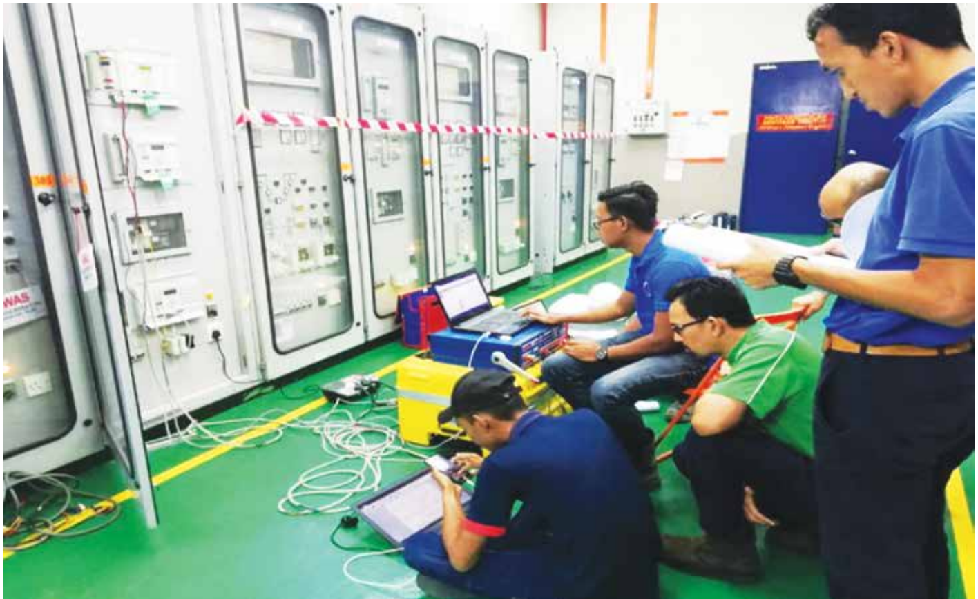
Service Engineers doing Relay Setting.
