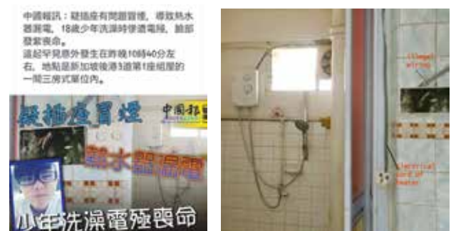
Figure 4: Case study of electrocution, where a new heater (with higher-rated power) was installed using the old method of installation, causing overheating of the socket, and resulting in an energized metal hose. Unfortunately, the user was electrocuted during the shower.
