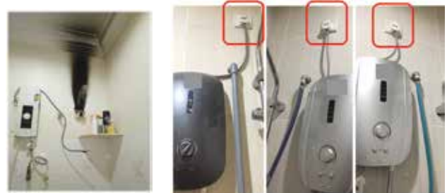
Figure 3: As seen in Malaysian homes, the instant water heater's electric power is connected from the 13A/15A socket outlet, in the shower cubicle, and it is used to run the heater with more than 15Amps supply. This is dangerous and overheating of the socket outlet is possible.
