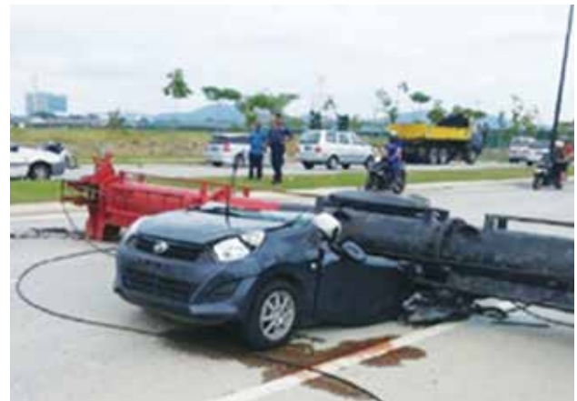
Gruesome sight! Heavy construction machinery collapsed and fell onto a passing car, instantaneously decimating two innocent occupants. It could have been us!
