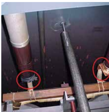
Figure 1: Base of two bushing connections (left side has coking, right side is OK)
