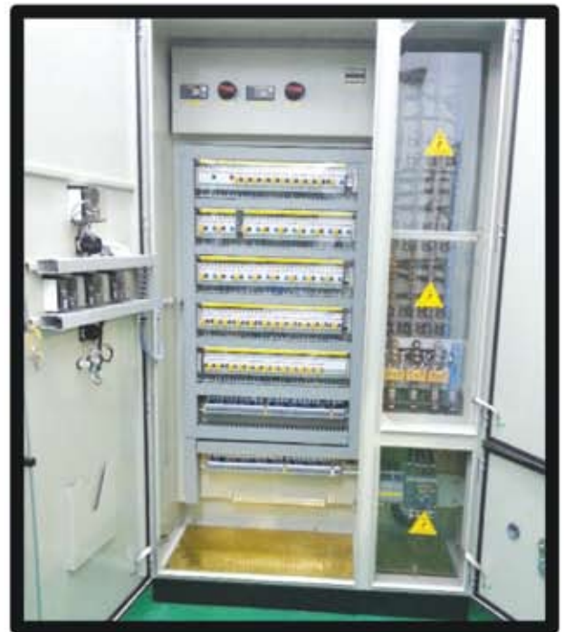
Electrical Distribution Board
