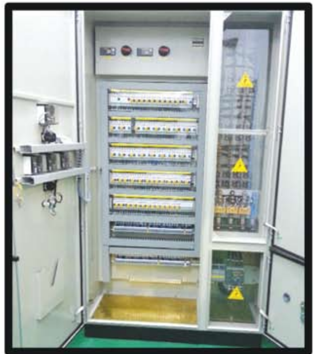
Electrical Distribution Board
