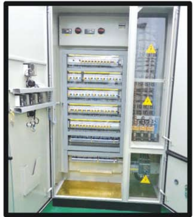
Electrical Distribution Board
