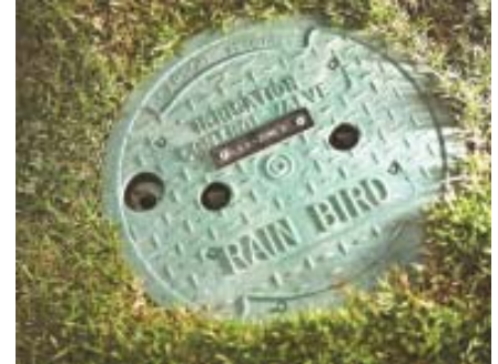
Irrigation control valve – Rain water that is harvested is controlled by this valve to the sprinkler system to irrigate the wetland.
