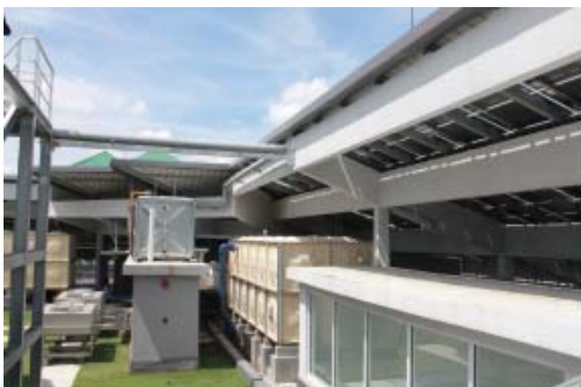
Solar panel installation – The diamond building was designed and built with the concept of a sustainable building with the installation of solar panel (on the right).
