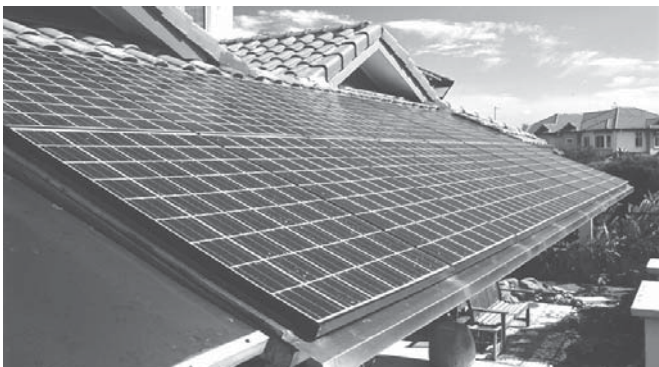
Source: Kota Damansara, 3.15 kWp, Selangor, Malaysia.
