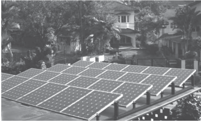
Source: Bukit Damansara, 4.2 kWp, Kuala Lumpur, Malaysia.
