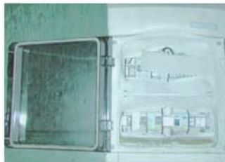
• Short circuit in the box due to internal contamination or humidity.
