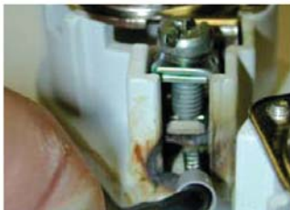
• Scorch mark due to loose clamping unit.
