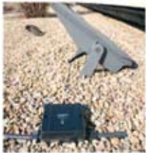
Unprotected outdoor installations which are close to the ground
