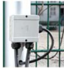
Ground-level unprotected outdoor installation
