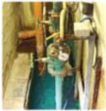
Pump shafts / stations
